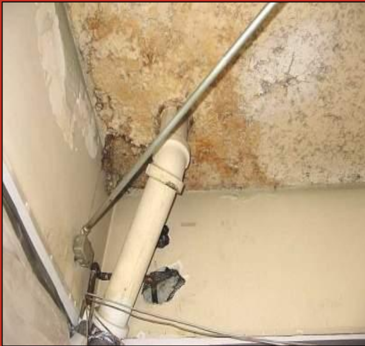
Water damage, deterioration
